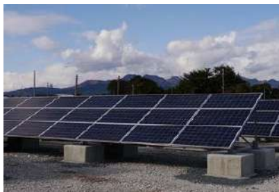
Hongo Photovoltaic Power Plant
