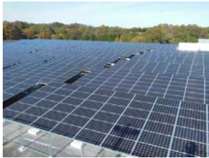
Elna Shirakawa Photovoltaic Power Plant
