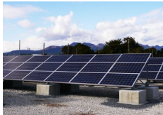
Hongo Photovoltaic Power Plant
