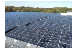
Elna Shirakawa Photovoltaic Power Plant
