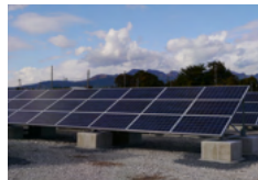
Hongo Photovoltaic Power Plant
