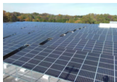
Elna Shirakawa Photovoltaic Power Plant
